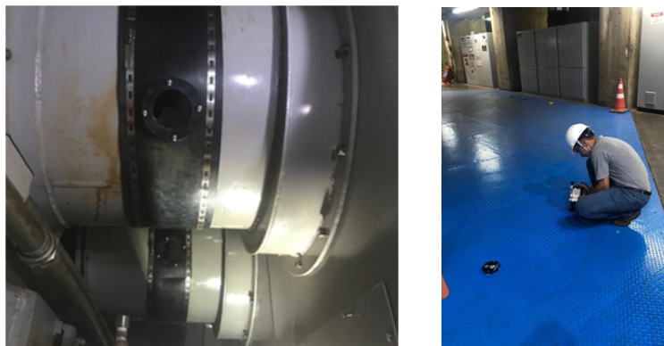
Example of installed windows for internal inspection of Barrel generator and pipeline connections (Image from JIT Brasil file).
