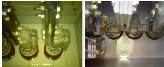
Examples of leaks in transformer bushings – inspection possible through windows with polycarbonate lids and glass lens (Images from JIT Brasil file).
