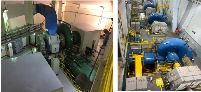
Example of PCH generators with windows installed in the generator connection boxes (Image from JIT Brasil file).
